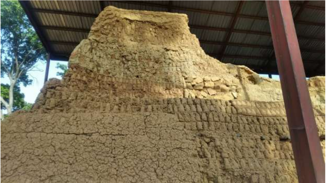
Figure 12: section of great wall of Kano with stacks of tubali under a canopy as conservation intervention
