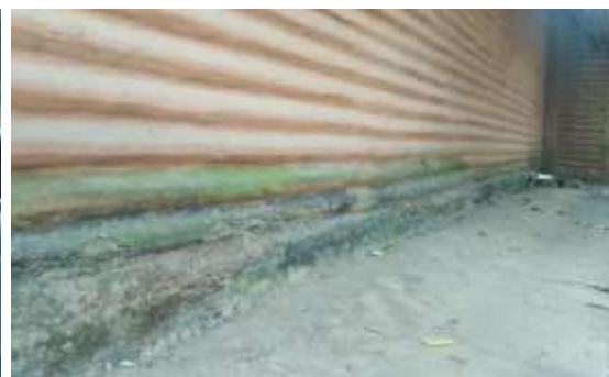
Figure 7: Mold on the base of exterior walls
