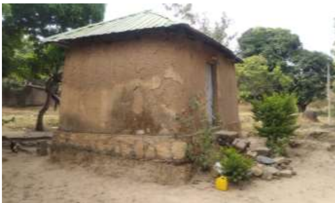
Figure 10: sole standing Irigwe hut in 2022 Dilapidated hut 2022
