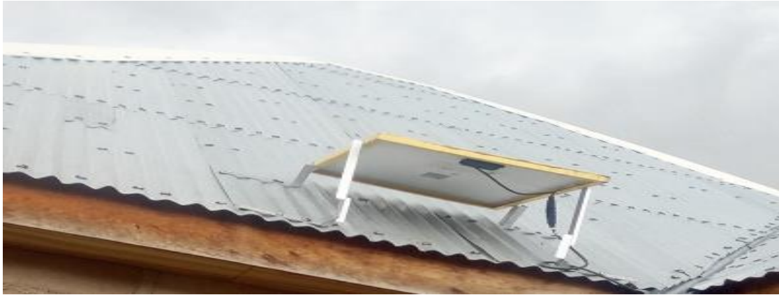
Plate 2: Showing the installation of solar panel on the roof of a building
