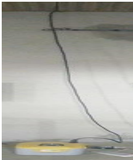
Plate 3: Showing the connection of a cable from solar panel connected to the MTN Lumos box.
