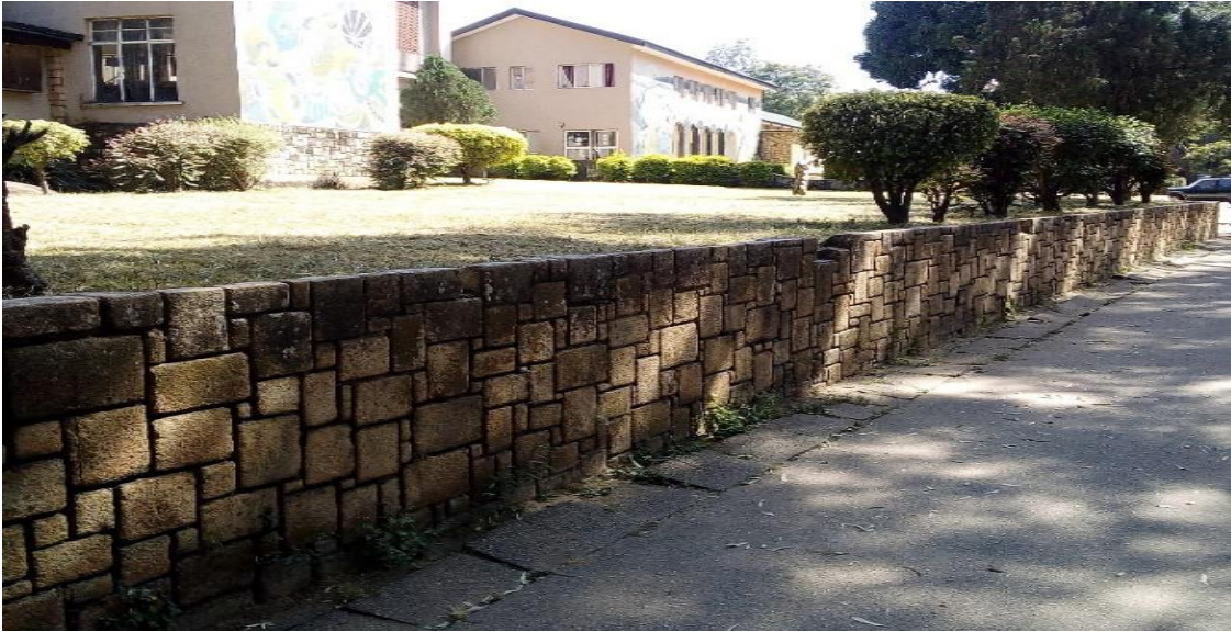
Plate iii: Retaining walls constructed from cut stones/ leading to the art gallery at Jos, Zoo building at the Jos Zoological Garden
